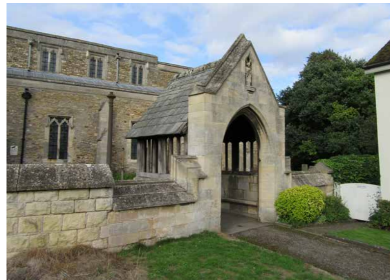
Fig 72: Attractive ashlar faced walling with moulded coping runs along the entirety of the churchyard frontage and is only interrupted by the ornate late 19th century lychgate, which forms a unique and charming gateway into the church grounds.
